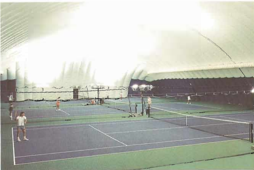
Interior view showing Zone-Controlled air ducts hung over player areas for maximum efficiency.
