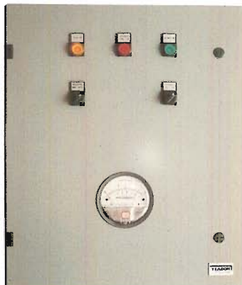
Wind Sensor Control Cabinet
